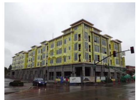
Under Construction 71 Unit - 4th & Main Apartments 4th Avenue and Main Street., Hillsboro
